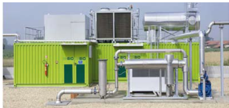
Parker Hannifin filter, cooler and condensate drain
